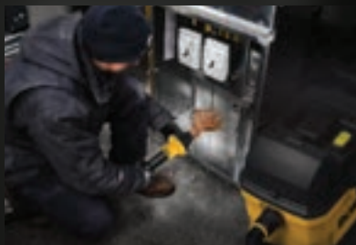
Multiple sizes of conduit for strong line-pulling suction
